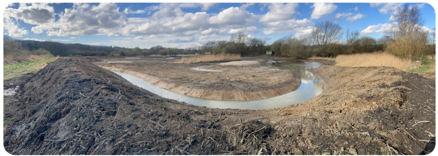
Work in progress to re-landscape Rodley Nature Reserve’s duck marsh, creating varied water depths and new banks to encourage greater diversity of wildlife
